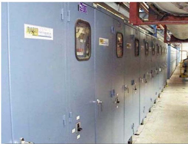
Continuous Tin Line Rectifiers
