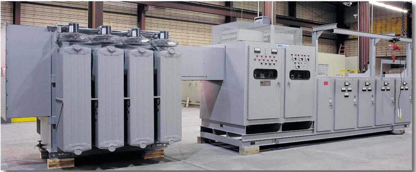
2,000 kW DC Substation
